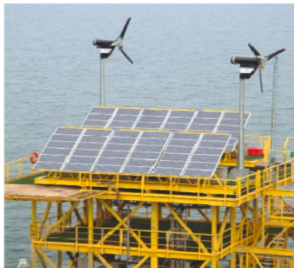
Fig. 1(a). Solar Powered offshore platform.
